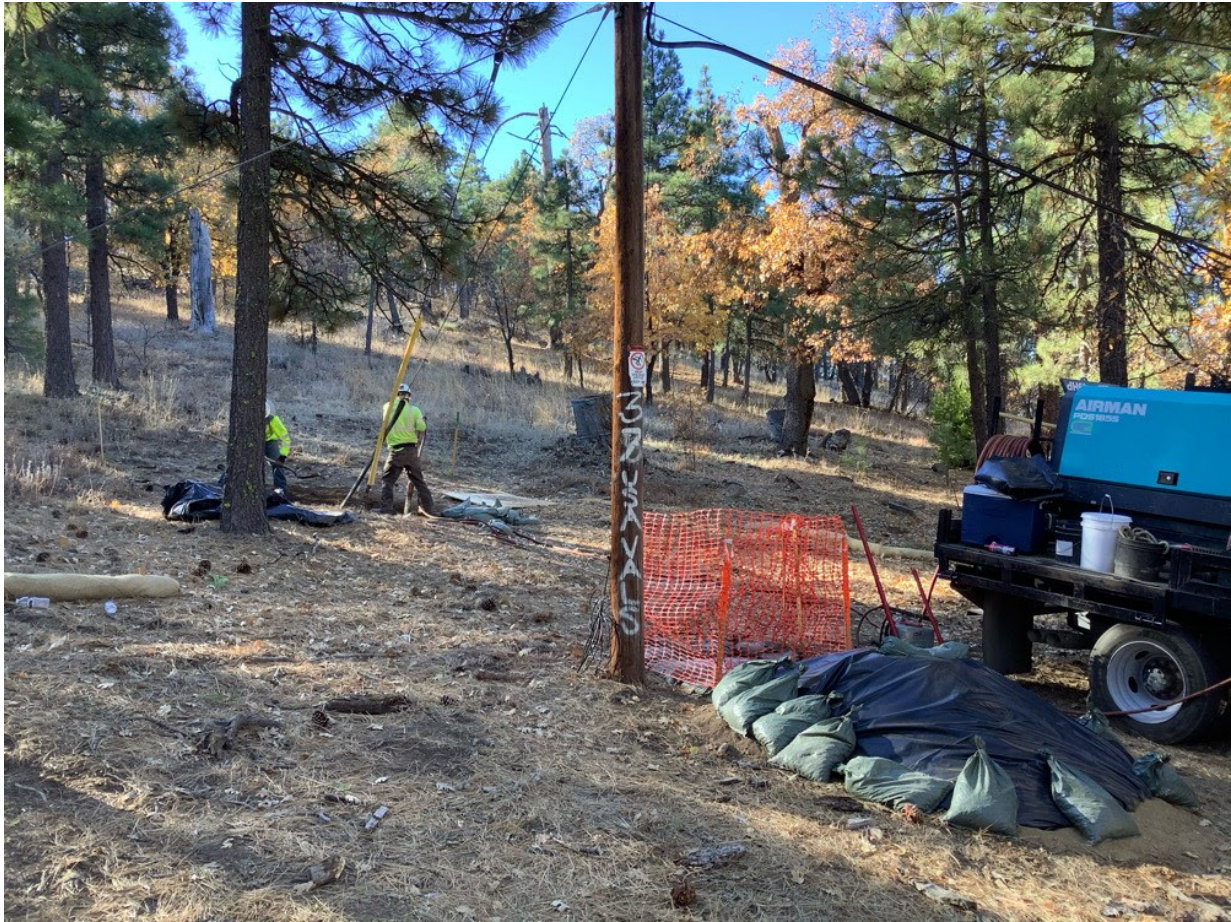
Photo 2: During anchor excavation at Pole P40354 (C 440), the pole hole was observed to be securely covered to prevent wildlife entrapment in accordance with MM BIO-23. Additionally, the associated spoils stockpile was observed to be covered in accordance with the ECP, the SWPPP, and APM HYD-09.
