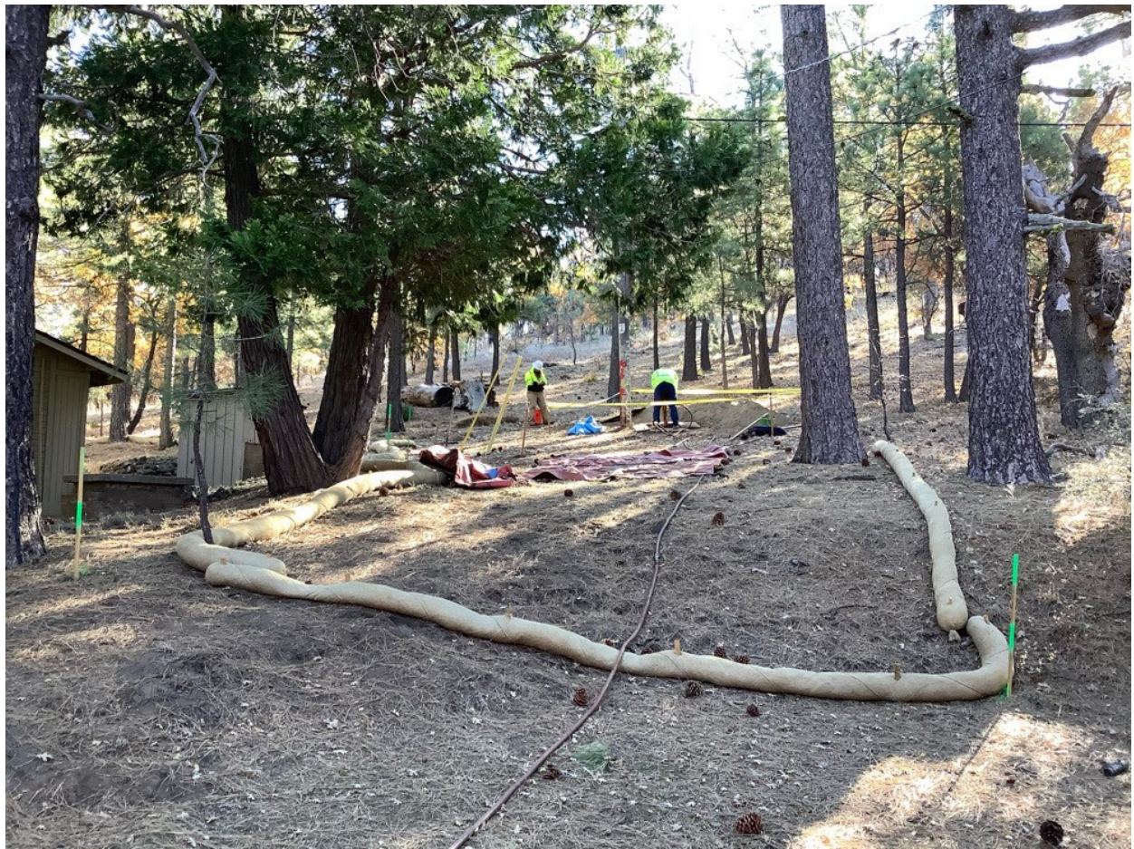
Photo 1: During pole hole digging at Pole P40352 (C 440), crew members and equipment were observed within clearly delineated work limits in accordance with MM BIO-1.
