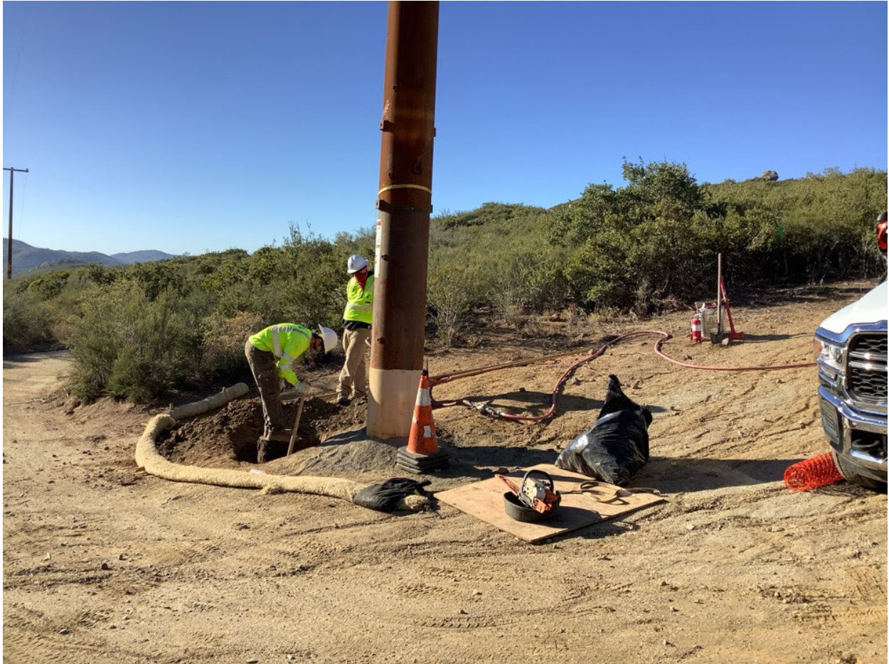
Photo 6: During pole butt removal at Pole P258545 (C 79B), a chain saw was observed to be staged in a drip pan to prevent leaks or spills from being discharged onto the ground in accordance with MM PHS-2 and the SRNP.
