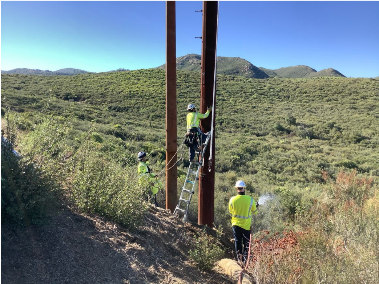
Photo 5: A Dedicated Fire Patrol was observed wetting the area prior to steel pole cutting at Pole P258494 (C 79B) in accordance with the CFPPP for hot work on NFS land with a PAL C.
