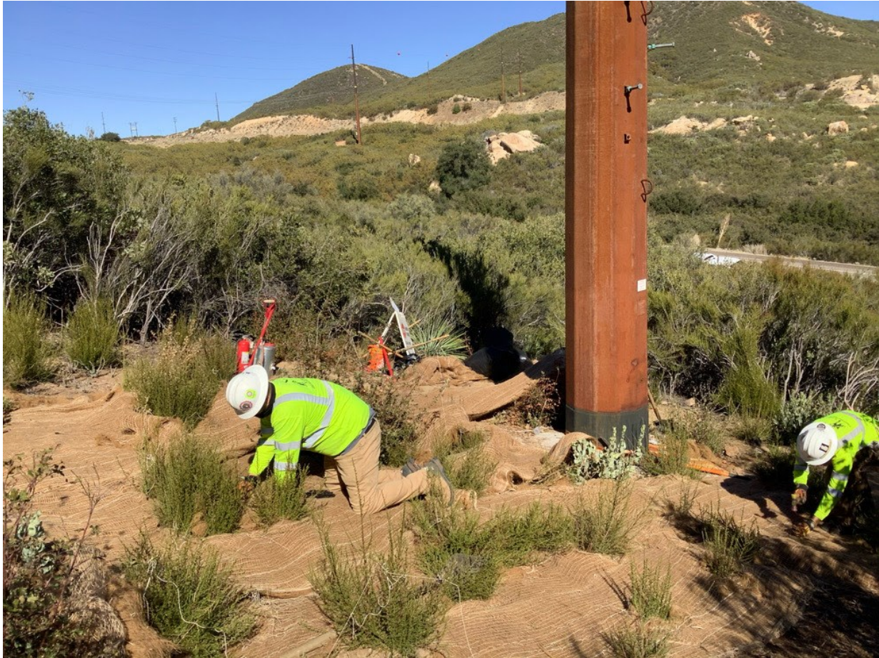
Photo 3: A crew was observed installing jute netting at Pole Z40256 (TL 629A) as part of habitat restoration activities in accordance with MM BIO-4 and the HRP.
