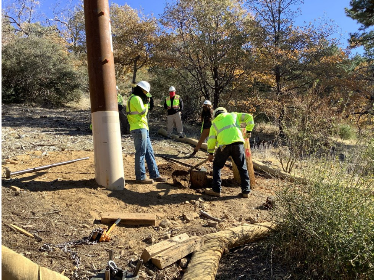
Photo 4: Archaeological and Cultural Monitors were observed monitoring pole butt removal on C 440 in accordance with the HPMP, MM CUL-1, MM CUL-3, and APM CUL-04.
